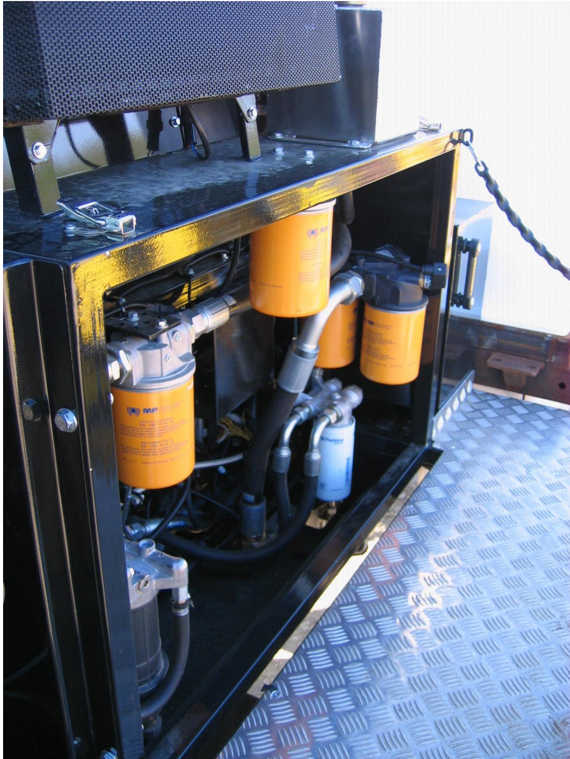
Figure 9 Filter Layout in Service Bay
